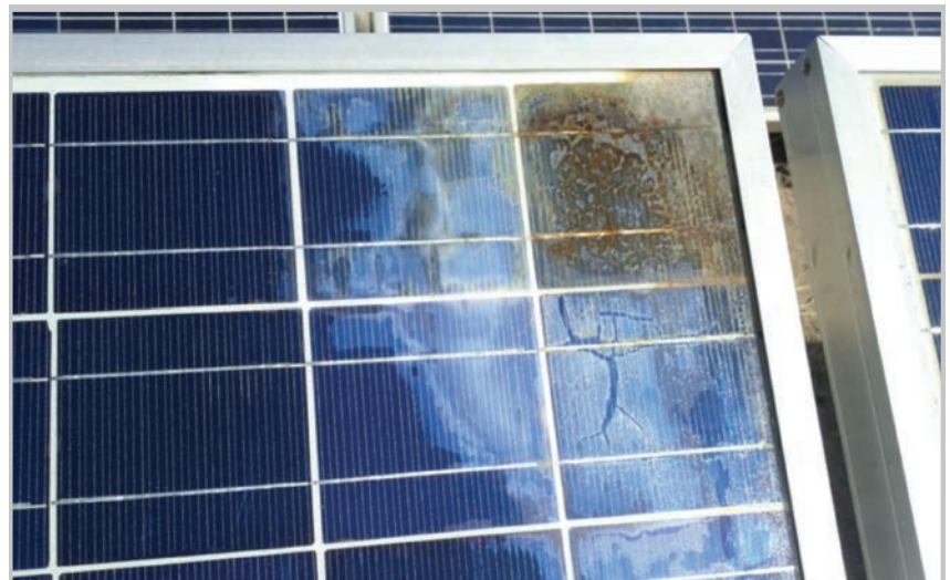
Damage such as that of the above panel can cause performance degradation and significant fire hazards
