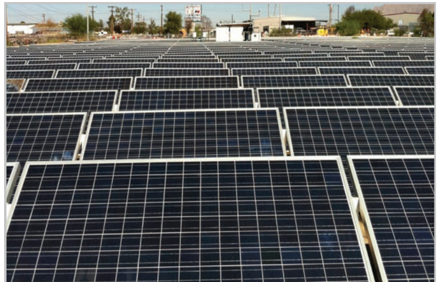
This large array in Tucson, AZ is the perfect test site for an optimizers retrofit
